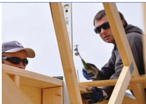
Lithuanian Construction Workers at a building site at Moss, Norway ©WPAINTSIL/IOM Oslo 2011
